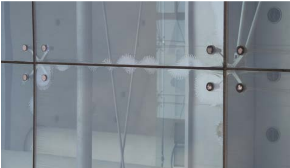
Typical defects caused by delamination.
